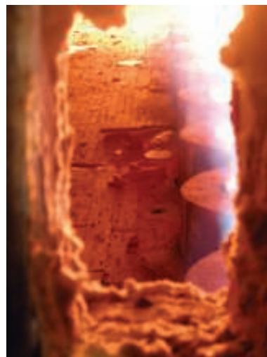
FIGURE 2. In this example of good troubleshooting, operators observed a failed tube hanger, which triggered the alarm for possible roof tubes sagging and led to the heater shut down for maintenance and hanger repair
