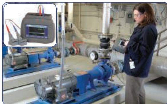
Verifying process flows with a Dynasonics DXN flowmeter (inset)
