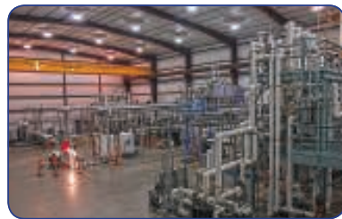
HTRI's research facility in Navasota, Tex.
