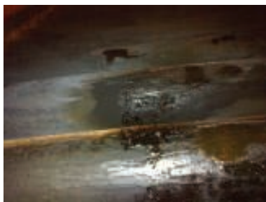
FIGURE 1. Misunderstanding warning signs led to a dramatic internal coke build up, followed by high tube metal temperatures, creep and finally tube rupture in one of the pass outlets of a visbreaker plant heater. Operators had unintentionally ignored high tube-skin temperatures for one week
